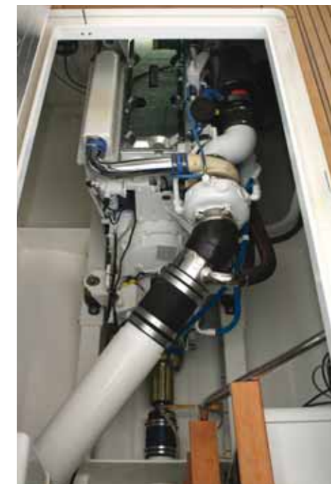
A fine example of a tidy engine room with good access
