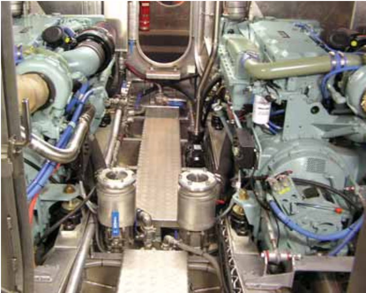
The engine room is busy but well laid out
